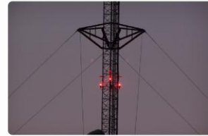
FAA RADIO TOWER LIGHTING
