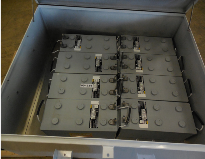
T-8X8D Enclosure with eight 8D batteries
