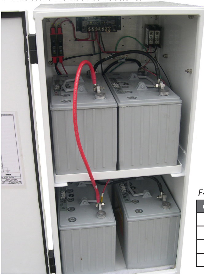
F4 Enclosure with four G31 batteries
