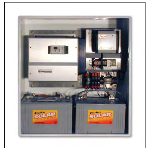
600 watt, 24V Power Online System
