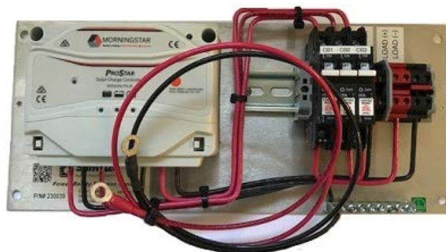
PRE Control Panel with a 30 amp ProStar
