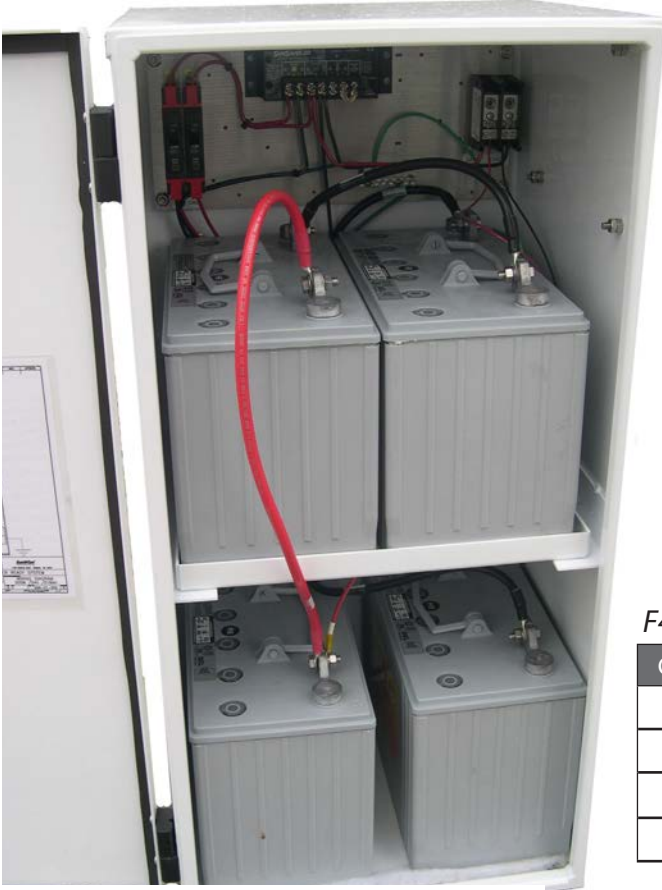
F4 Enclosure with four G31 batteries
