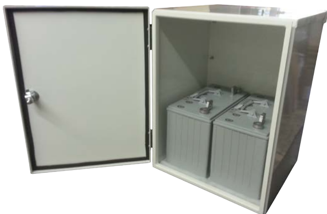
F2 Enclosure with two G31 batteries
