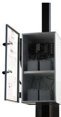
Pole Mounted, SWPB Power Online System
