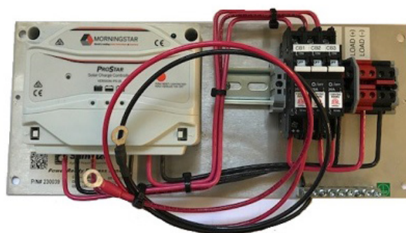
PRE Control Panel with a 30 amp ProStar
