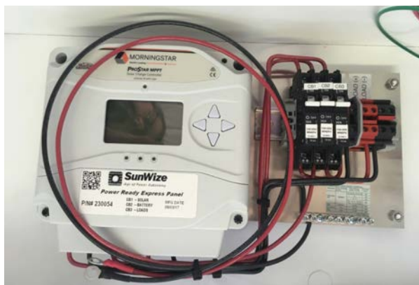
PRE Control Panel with a 25 amp MPPT ProStar w/ meter
