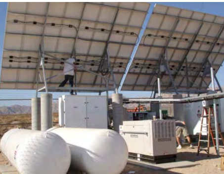
Solar & Generator Hybrid Telecom System 2
