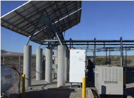
Solar & Generator Hybrid Telecom System 1
