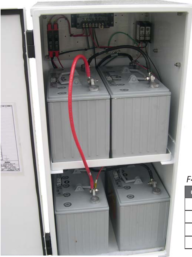
F4 Enclosure with four G31 batteries
