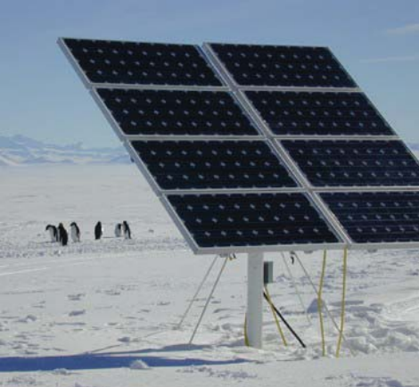
SunWize® Power Ready System in Antarctica.
