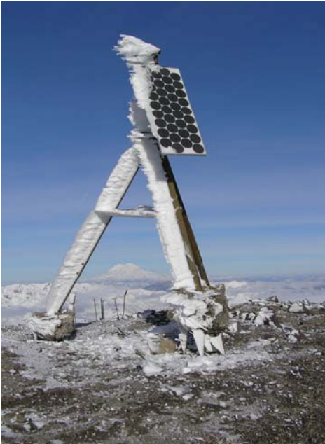
A SunWize® Power Ready System exposed to severe weather on Mt. St. Helens, WA. The system powers a camera that takes photos of the lava dome.
