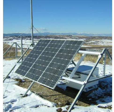
A SunWize® Power Ready System in Castle Rock, CO powering a 2.5 amp, 12VDC remote telemetry unit.
