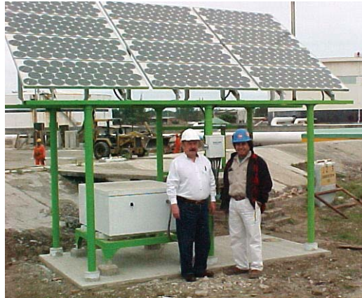
SunWize® Power Ready System providing power for oil and gas pipeline monitoring equipment.
