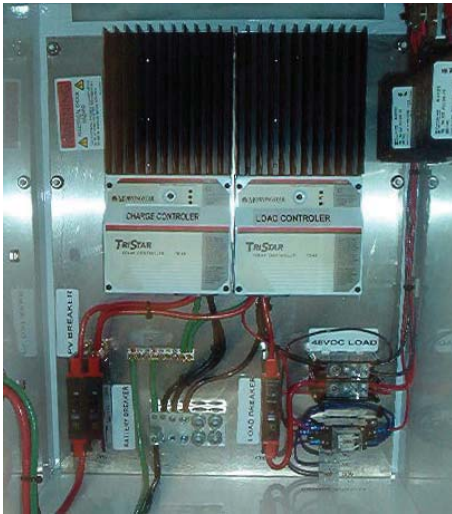
PV controller, load management controller and LVA in an aluminum enclosure.
