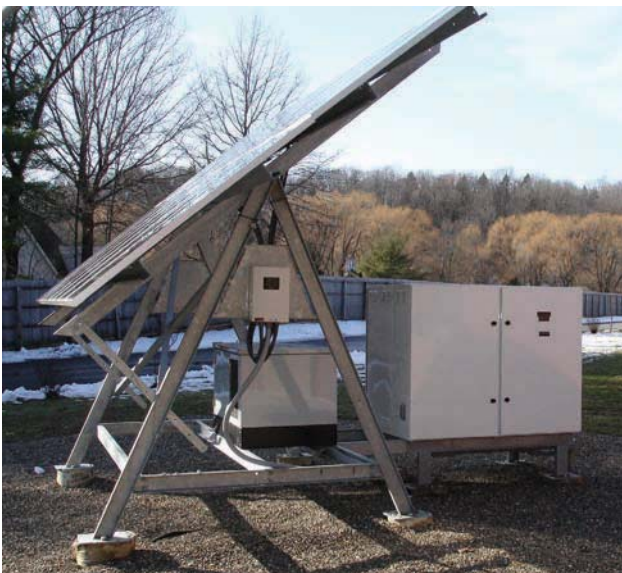
SunWize® Power Station
