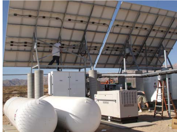
The back of a SunWize® Power Station solar array showing generator and propane tanks powering 2 BTS radios and a microwave radio in California.
