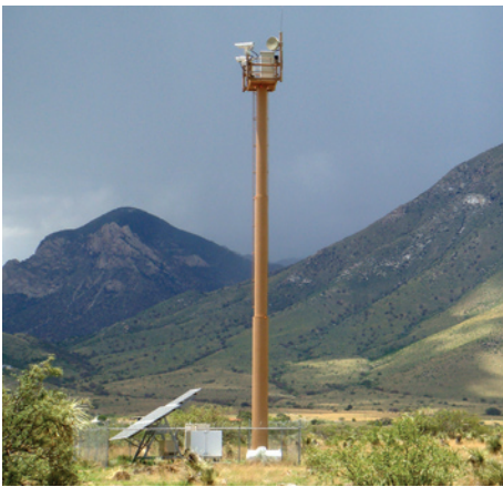
SunWize® Power Station
